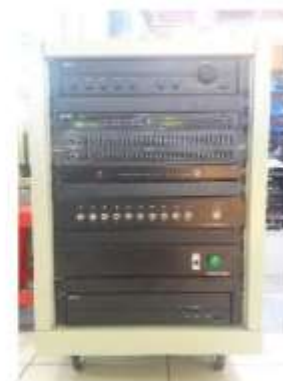
Public Address System (PA System)
