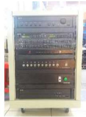
Public Address System (PA System)
