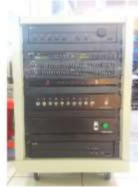
Public Address System (PA System)
