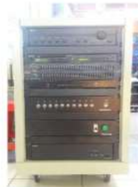
Public Address System (PA System)
