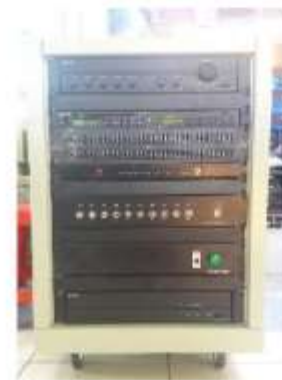
Public Address System (PA System)
